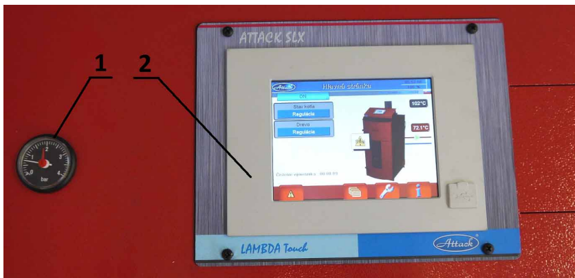
Figure 16 1 – manometer, 2 – touch screen
