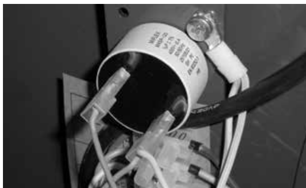
Location of the starting capacitor (1µF) for an exhaust fan
