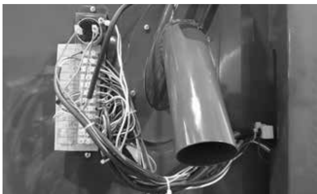
Electrical installation of the boiler under the front bonnet
